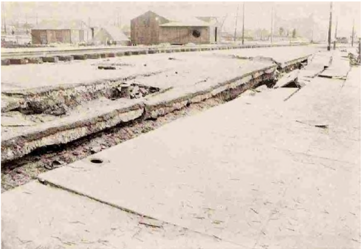
Effects of Shock: Separation of the Sidewalk from the Asphalt Paving on Capp Street, Between Seventeenth and Eighteenth Streets.
