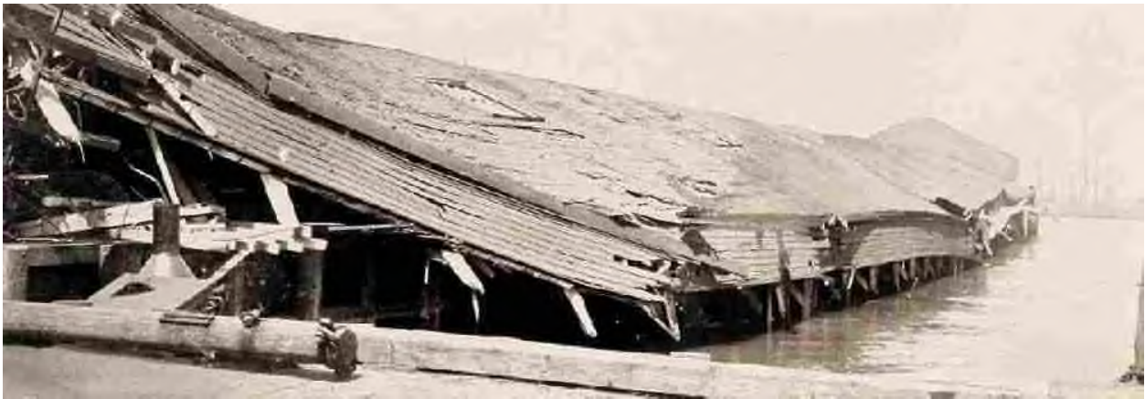
Effects of Shock: Collapse of Wharf No. 7, Near Ferry Building.
