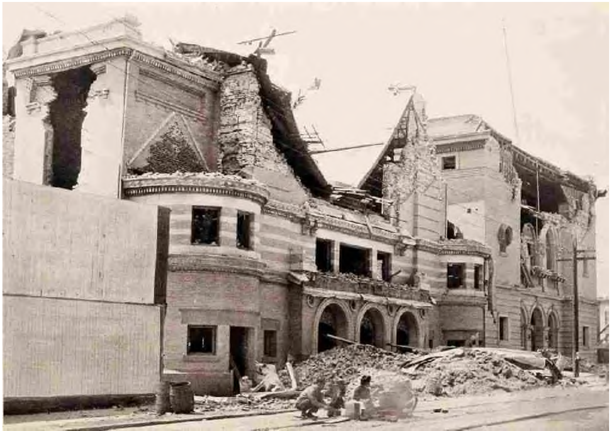
Effects of Shock on Newly-Constructed Temple Beth-Israel, 1817 Geary Street, Western Addition.
