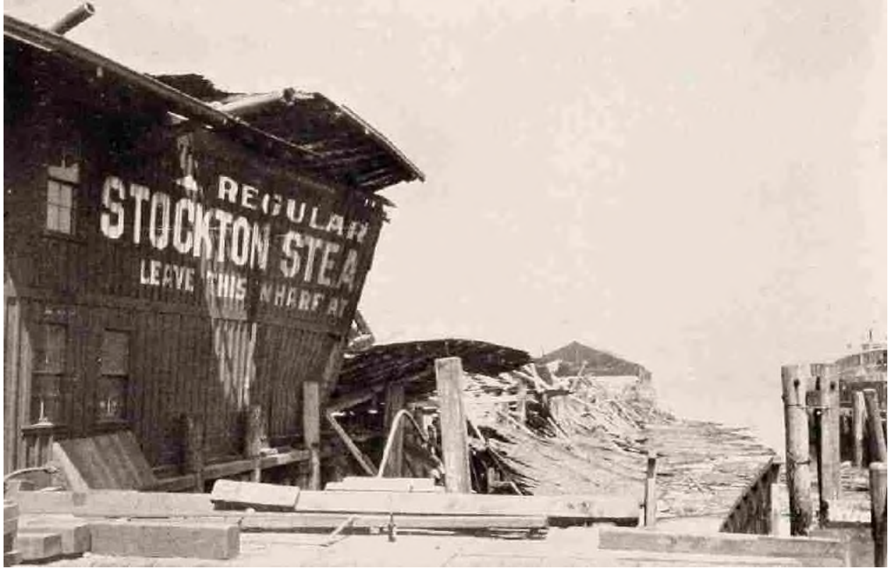
Effects of Shock: Collapse of the Stockton Steamer Wharf, Water Front, Near Ferry Building.
