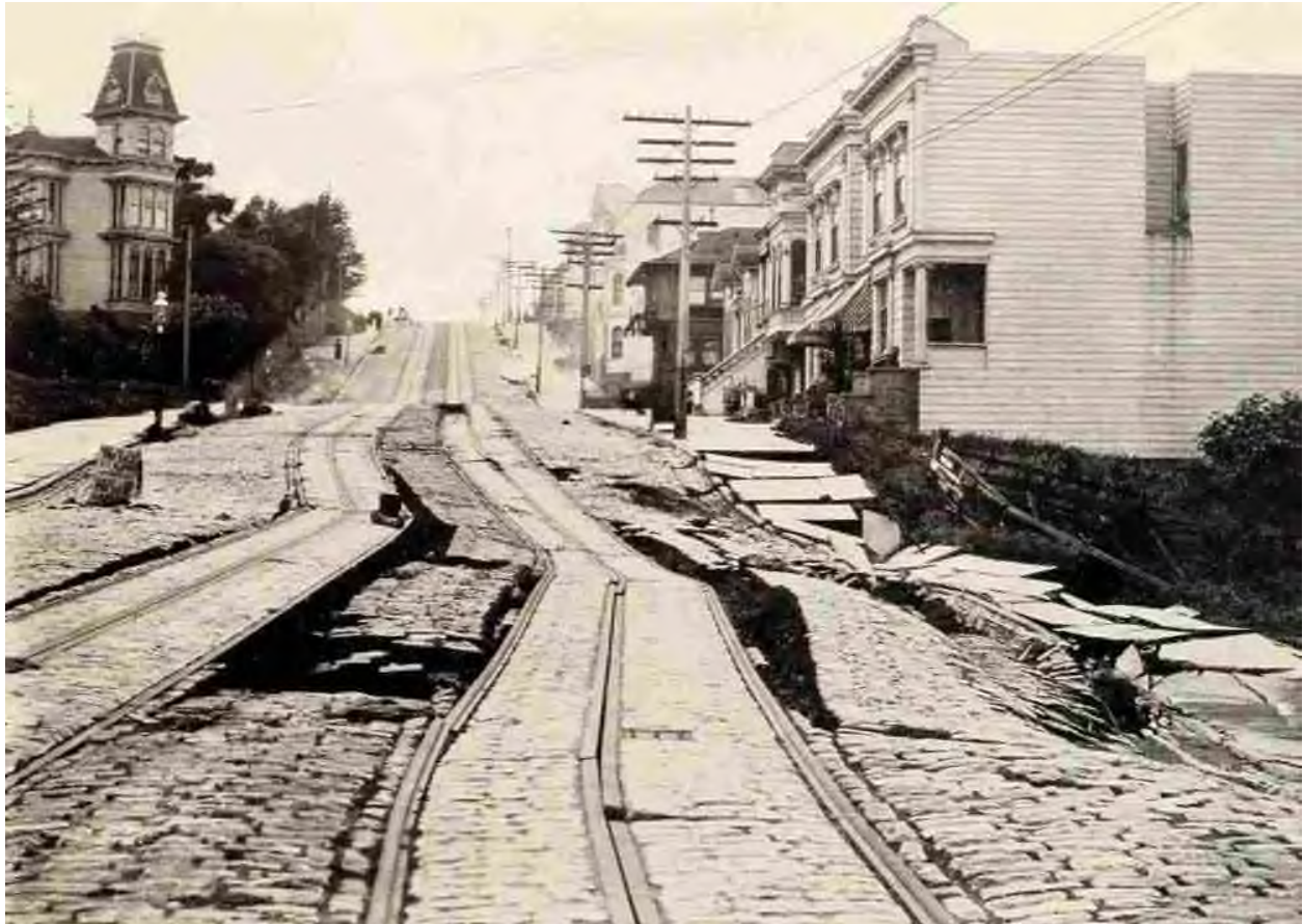
Section of the Union Street Cable Line, Between Steiner and Pierce Streets, Distorted by the Earthquake.
