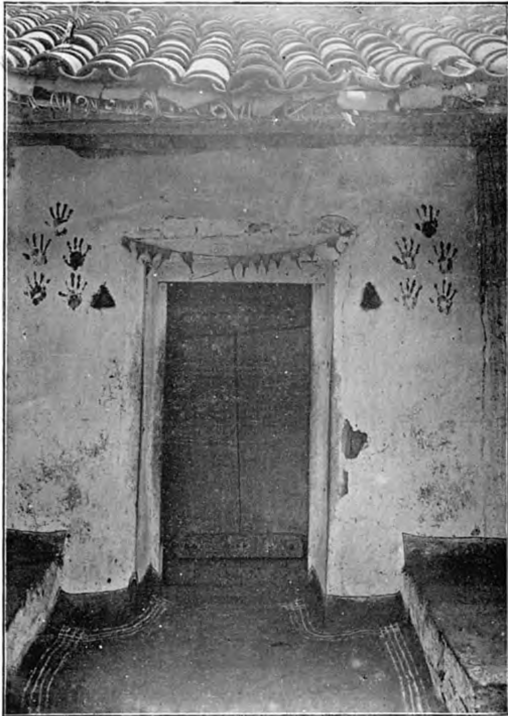
Brāhman House with Marks of Hand to Ward Off the Evil Eye.
